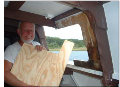
A bothersome window leak turned out to require replacing a whole section of wall
